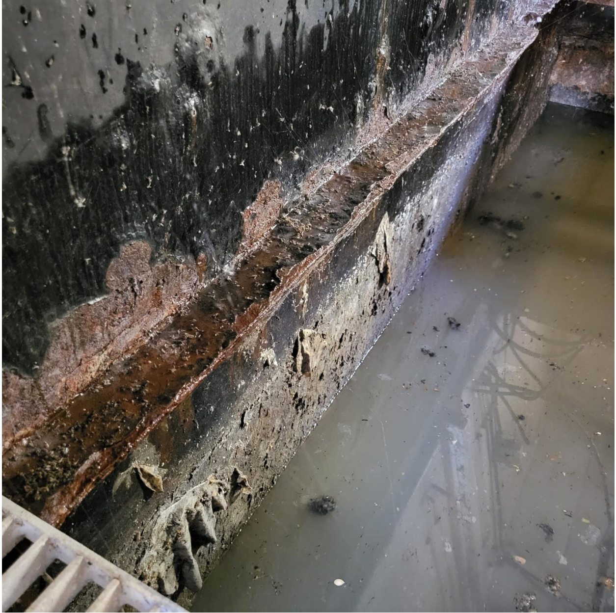
Corrosion in primary clarifier chamber of outer tank
