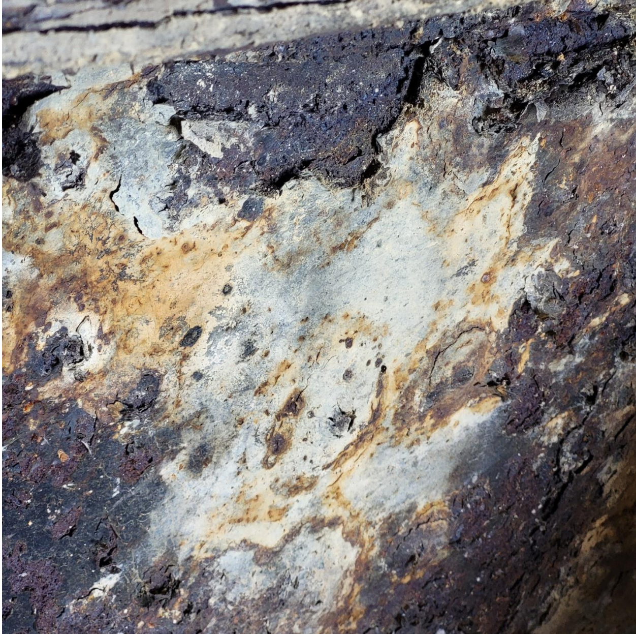
Biozone tank end wall corroded
