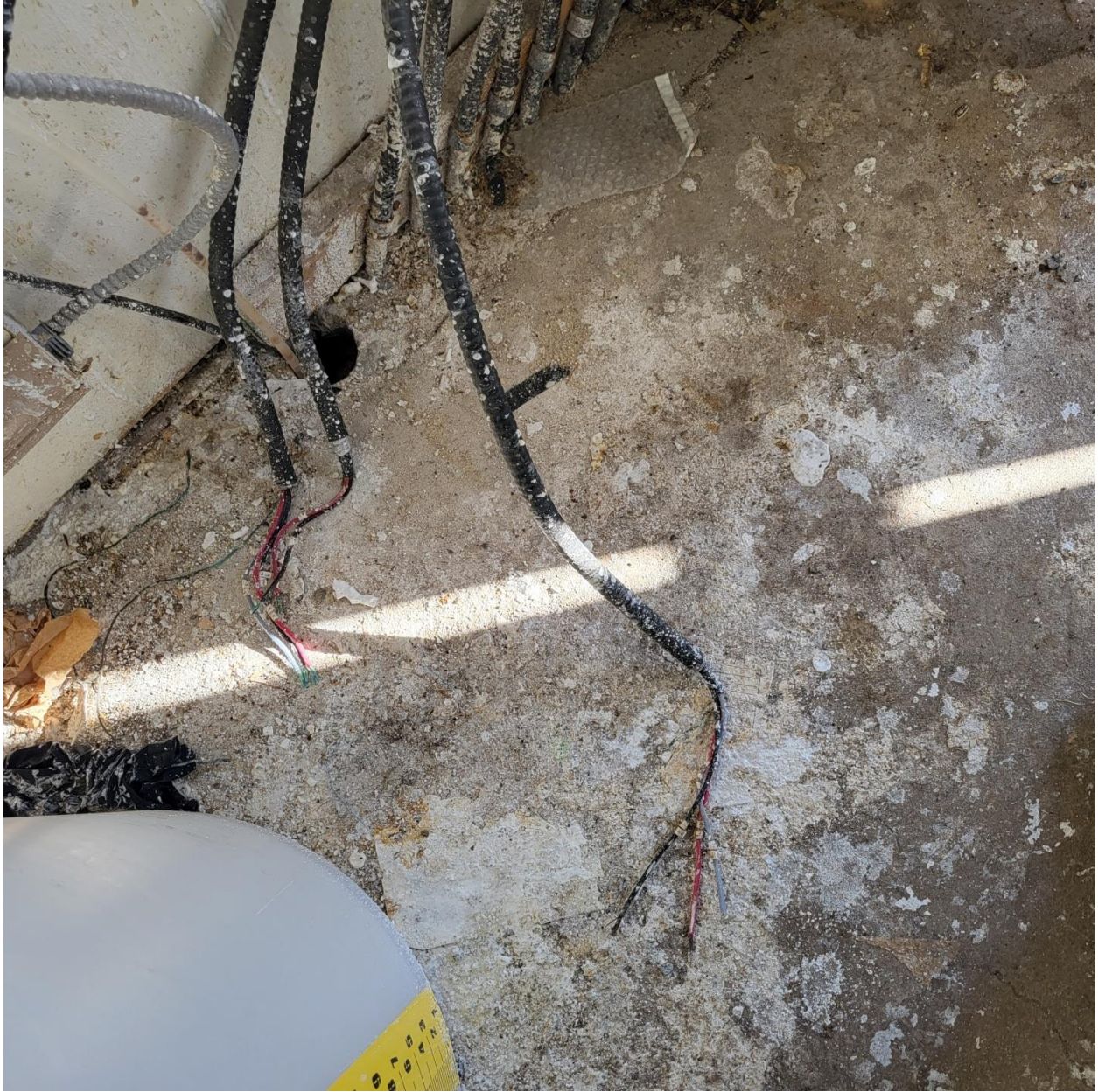
Disconnected wiring in control room
