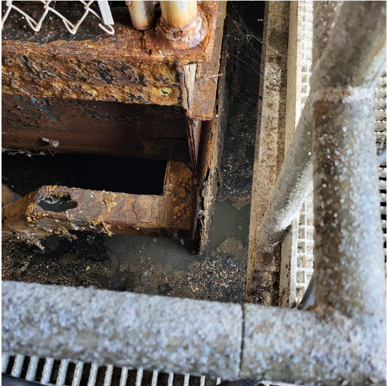
Drive end corner of biozone on left when facing RBC module shows significant corrosion
