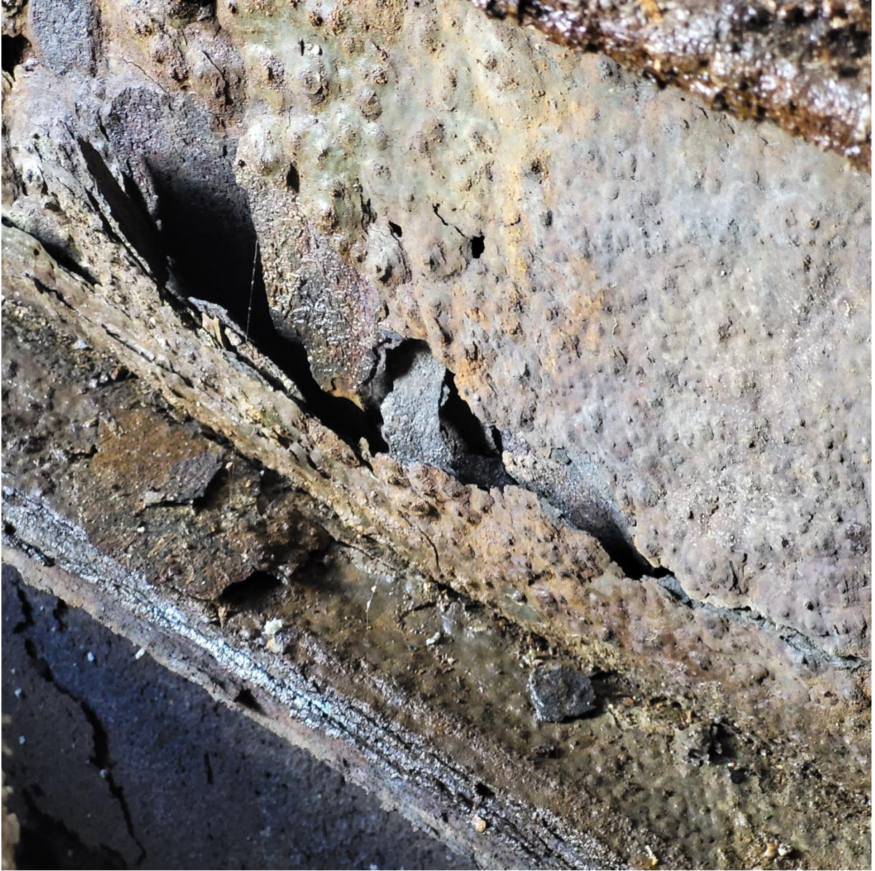
Biozone tank side wall shows significant corrosion
