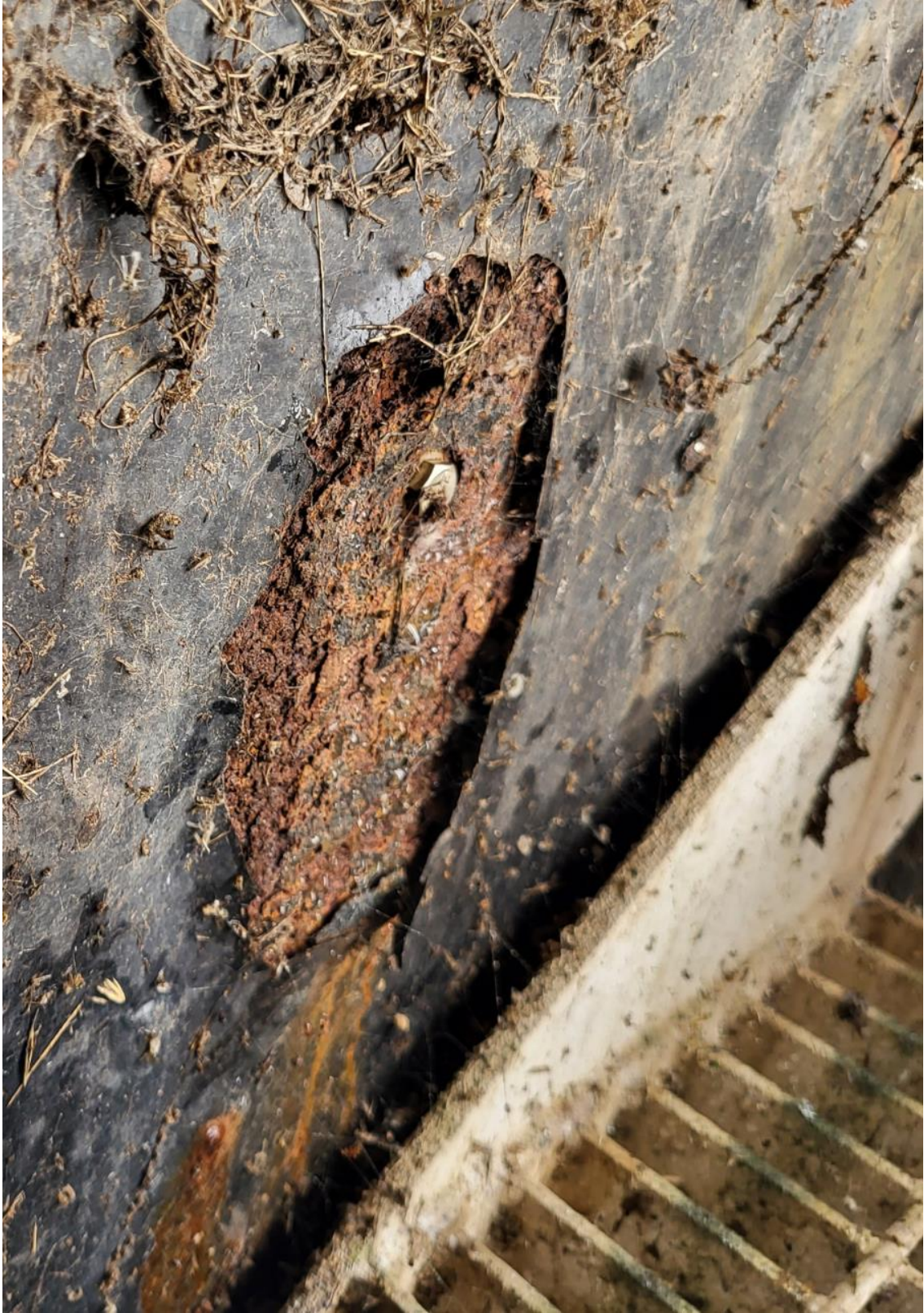
Corrosion of outer tank at stainless steel fastener
