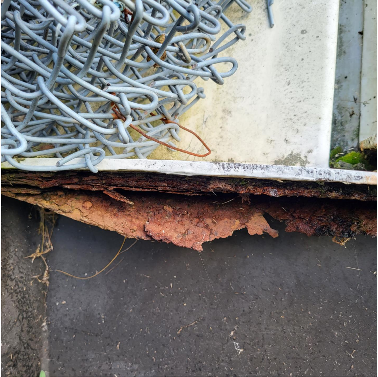
Corrosion of outer tank lip immediately below FRP cover on south side of outer tank
