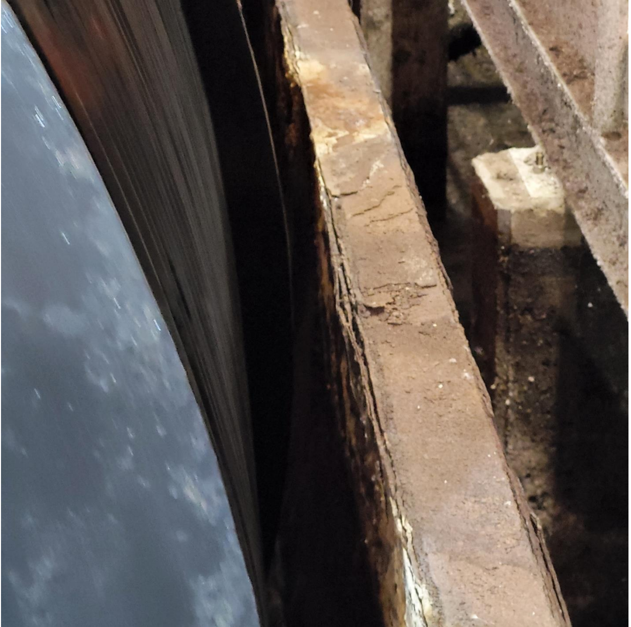
Biozone tank lip rail support corroded
