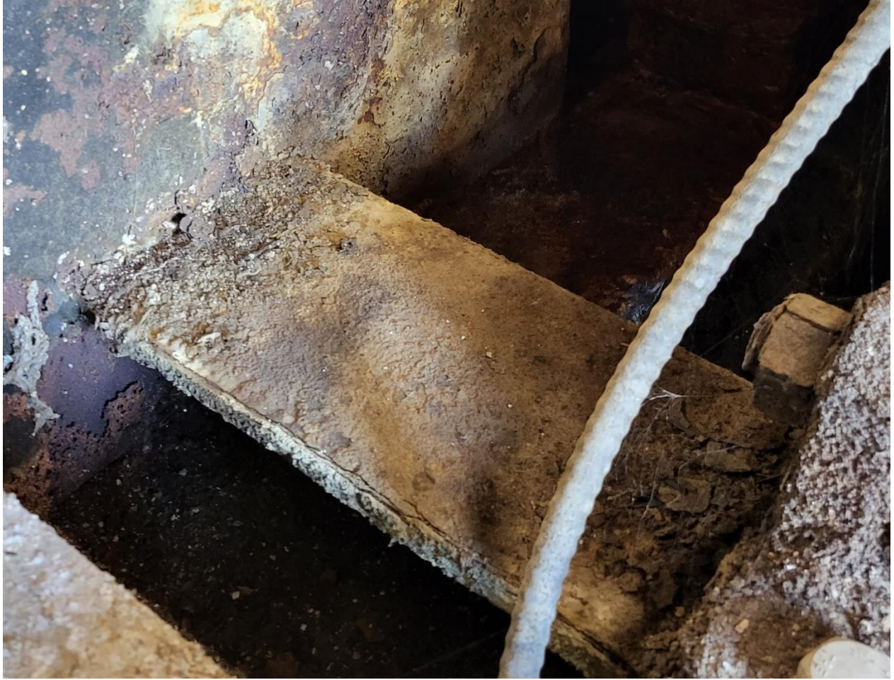
Torque arm support corroded
