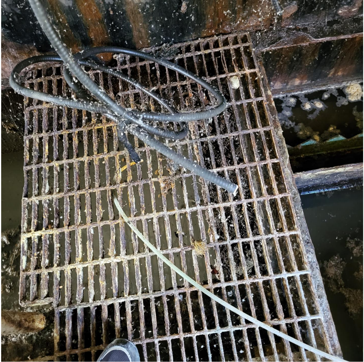
Disconnected wiring in treatment tank
