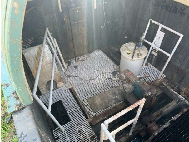
Figure 2-7: Aluminum Grating Platform
