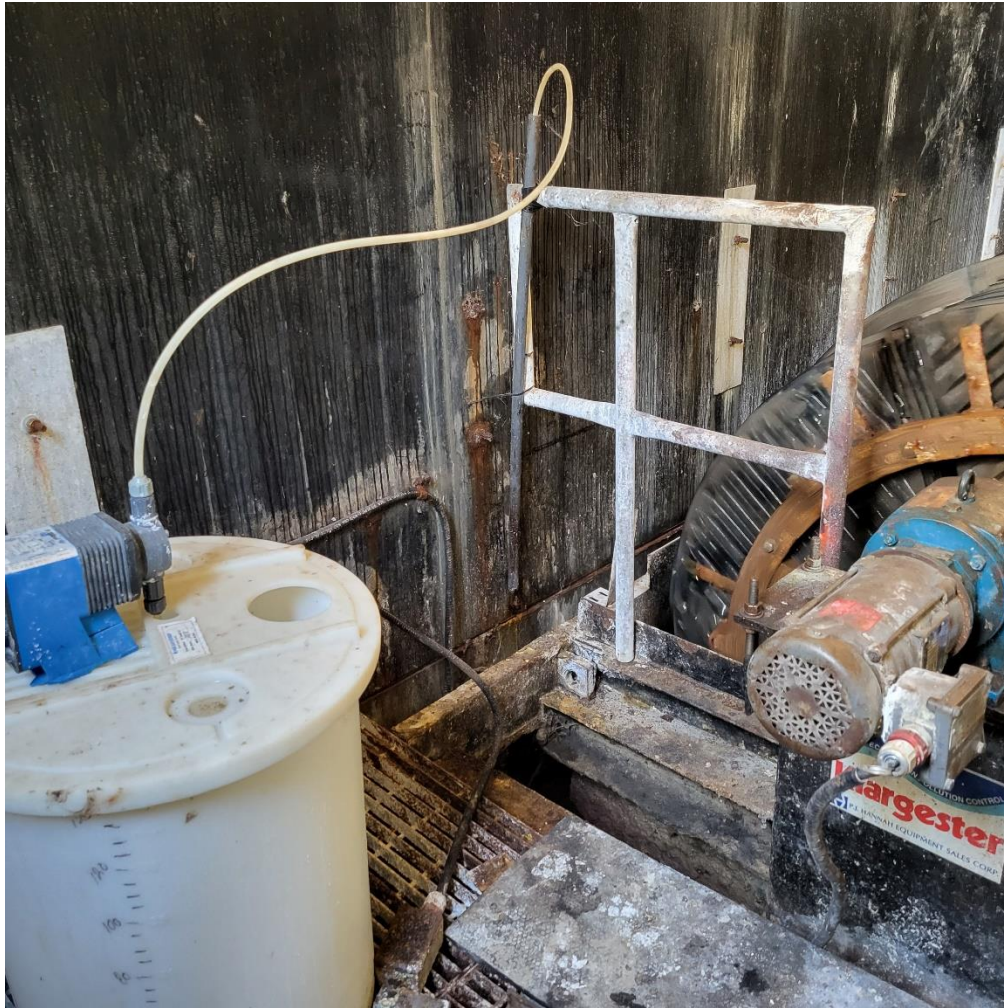
Alum dosing system and injection point.
