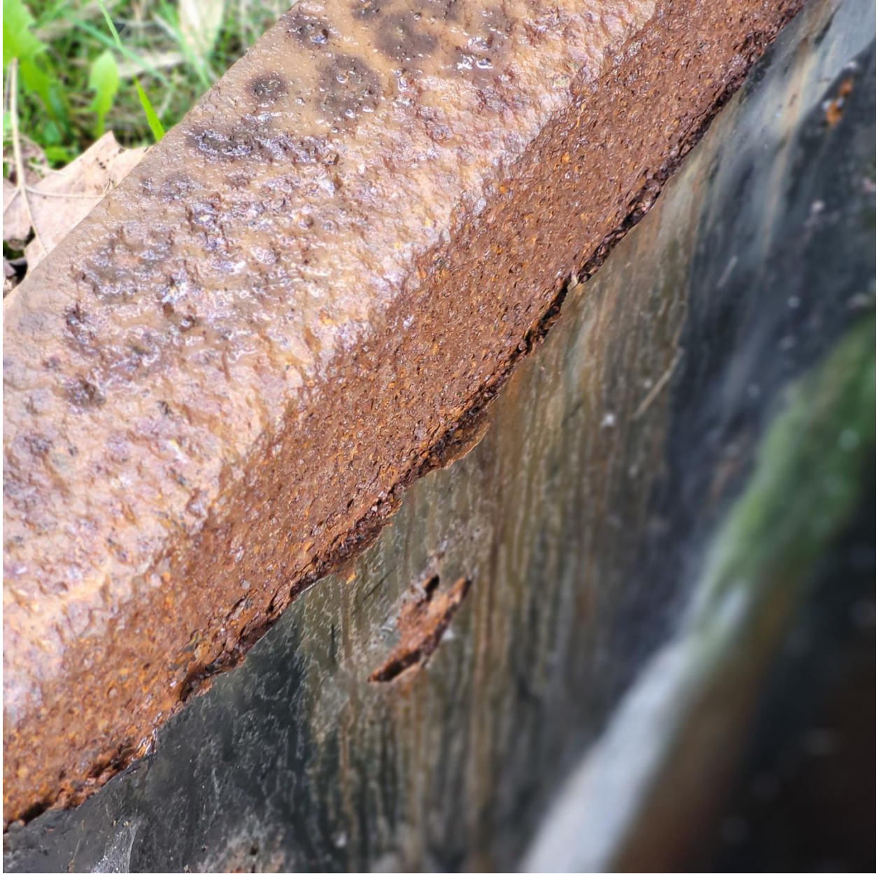
Corrosion on lip of outer tank at access hatch
