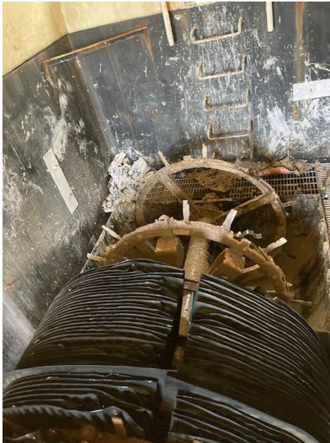
Bank one failure fall 2023
