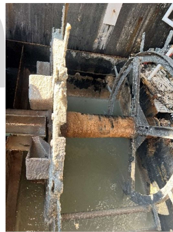
Figure 2-6: Corroded Shaft Bearing
