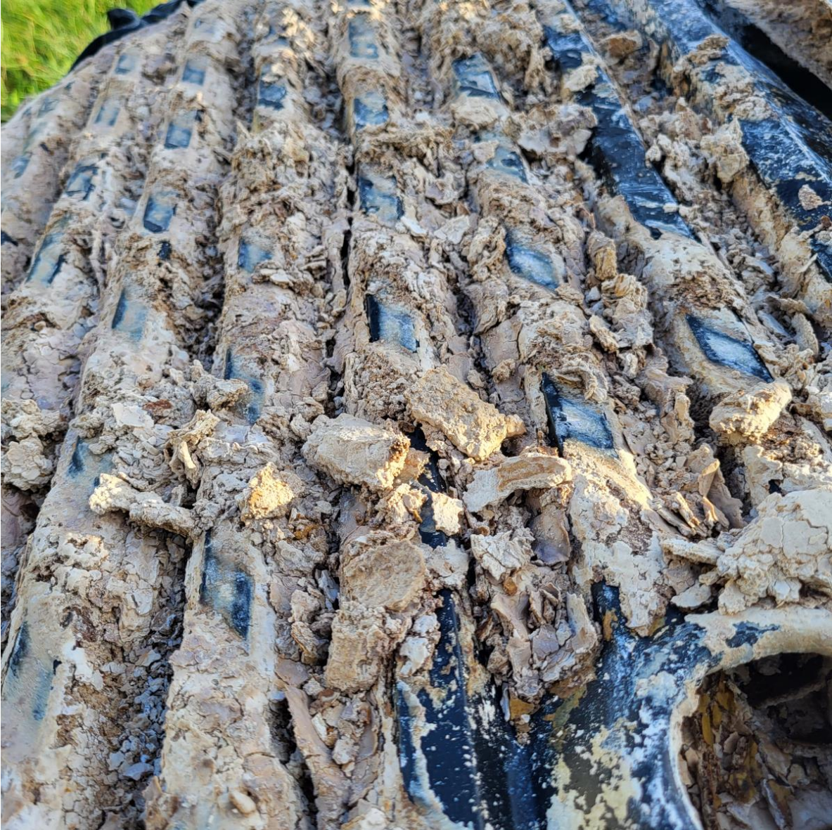
Very heavy alum build up is evident on discarded media sheets from bank one.
