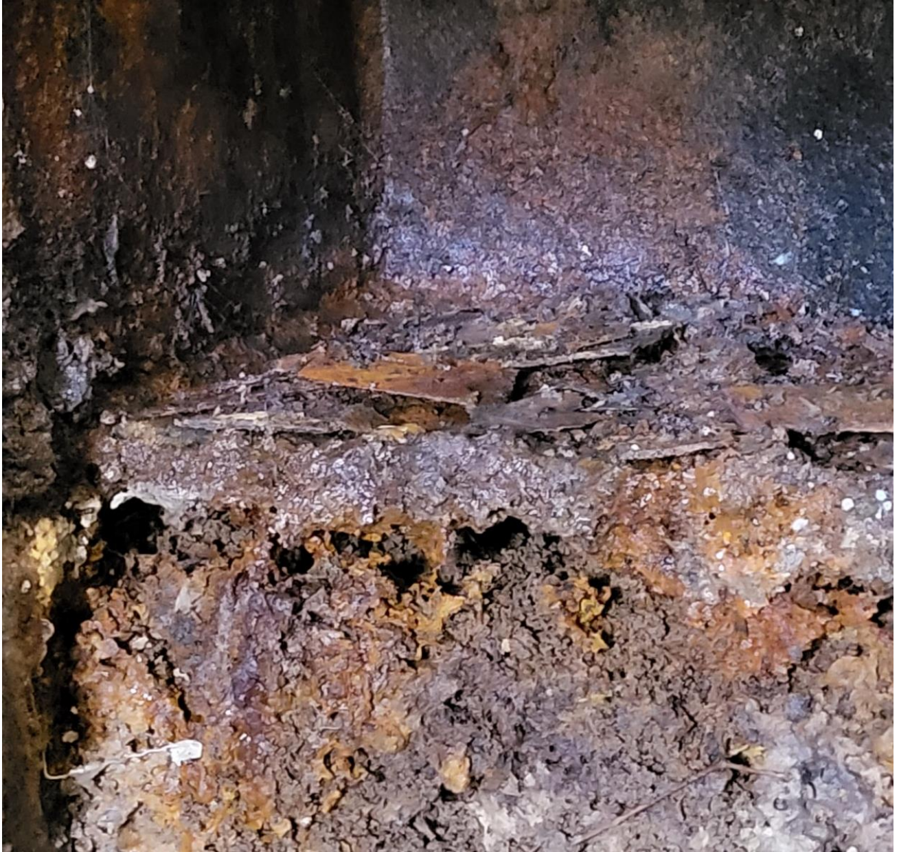
Corrosion of outer tank near alum feed line
