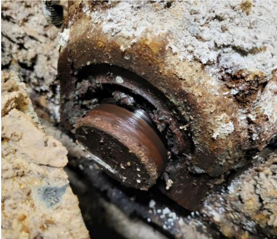
Failed bearing should be replaced
