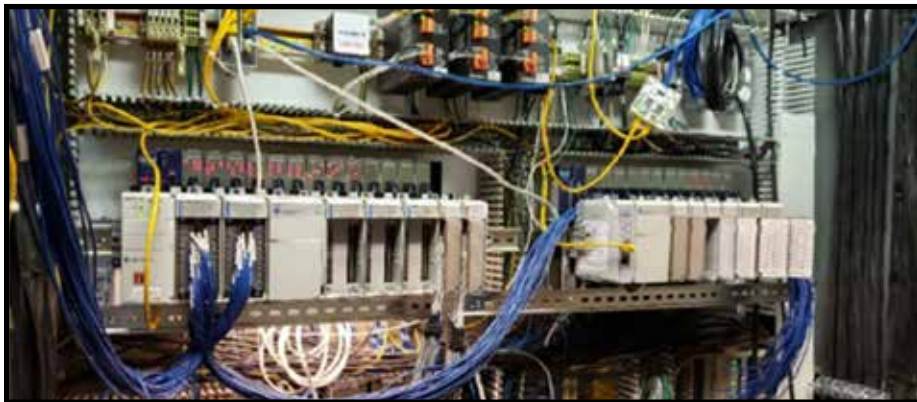
Electrical Room SCADA Panel Controllers
